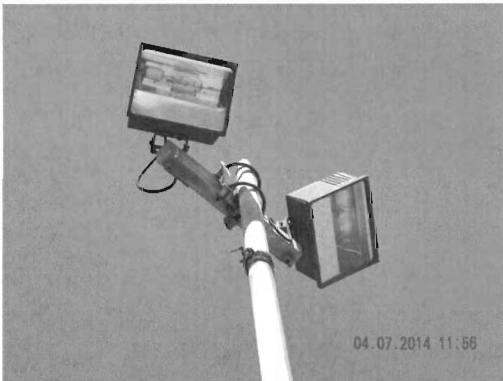
City of Monterey Park Existing Light Fixtures at Parks
