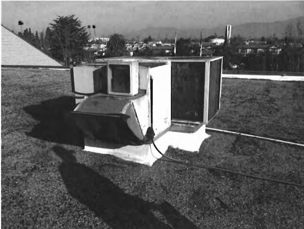
City of Monterey Park Existing RTUs at City Hall
