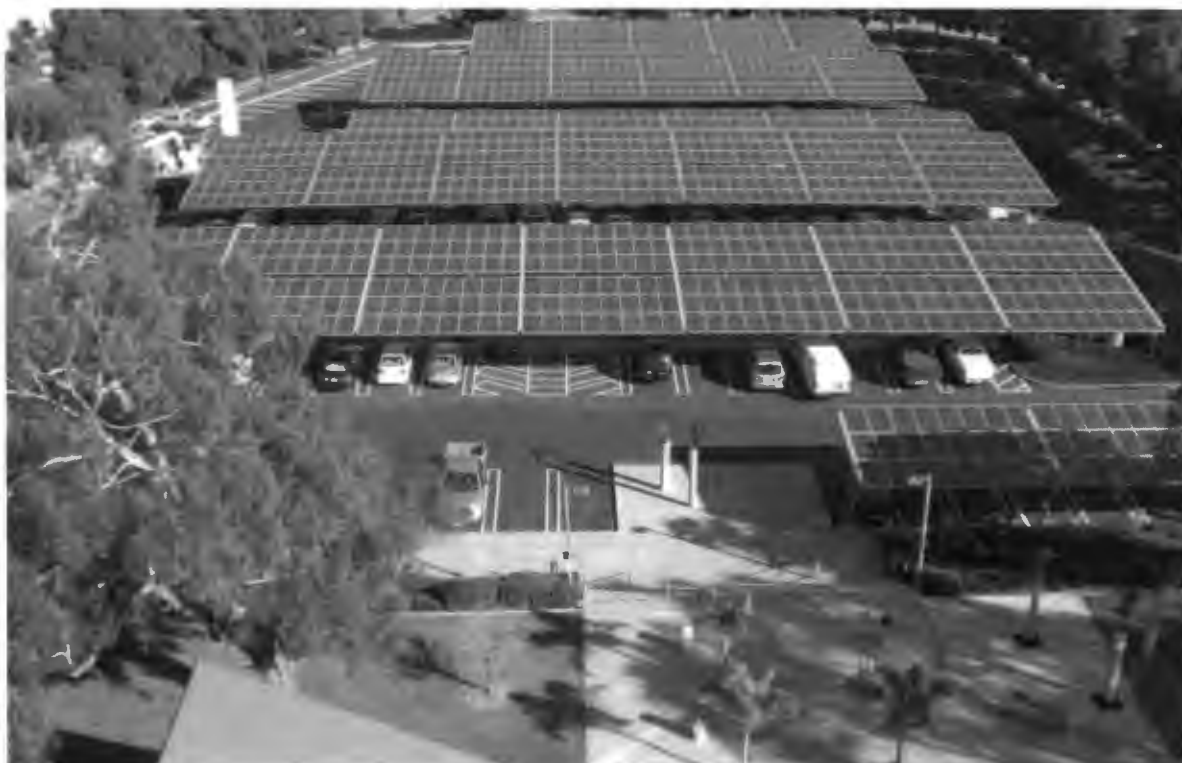
Figure 4: One of SunEdison's solar canopy systems at the City of Huntington Beach.
