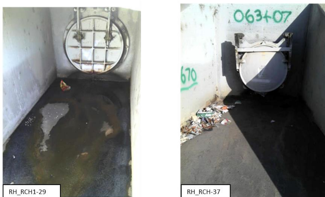
Figure 7.5. Outlier outfalls RH-RCH1-29 and RH-RCH1-37 (Lower LA River WMP Group).
