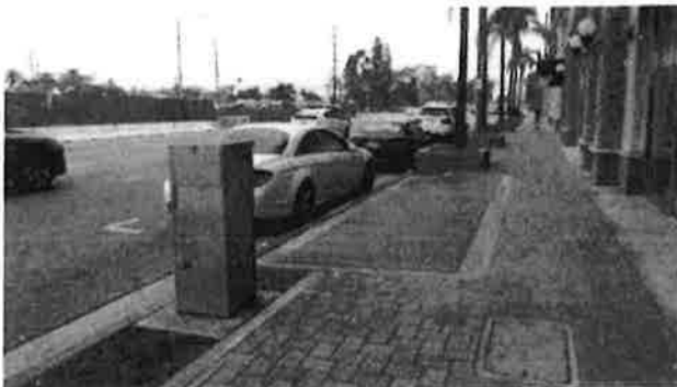
PHOTO 3: UNDERGROUND UTILITY VAULT ON SIDEWALK
