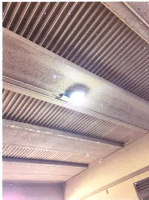
Figure 4 – Ceiling mounted LED light fixture
