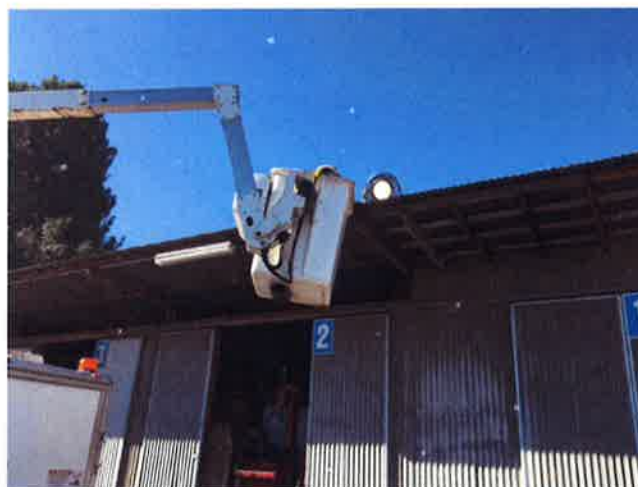
Figure 8 – Exterior LED Flood Light
