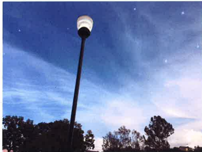
Figure 7 – Exterior Pole Light
