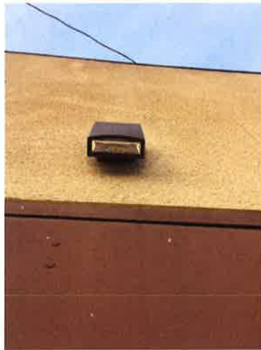
Figure 6 – Exterior Wall Pack
